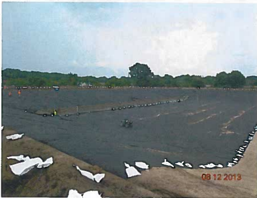
Extent of work completed on Day 1, south end of basin (looking southeast)
