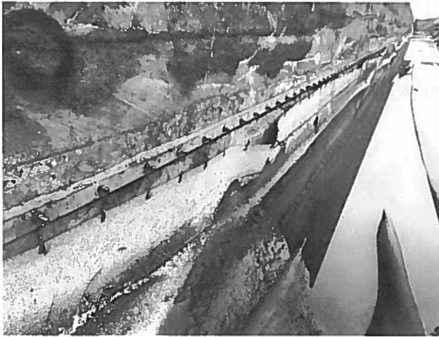
Damaged connection to batten strip on north side of weir wall, facing southwest
