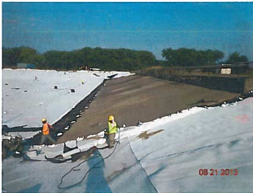
Extent of geosynthetic deployment on the south end of the basin (looking east)
