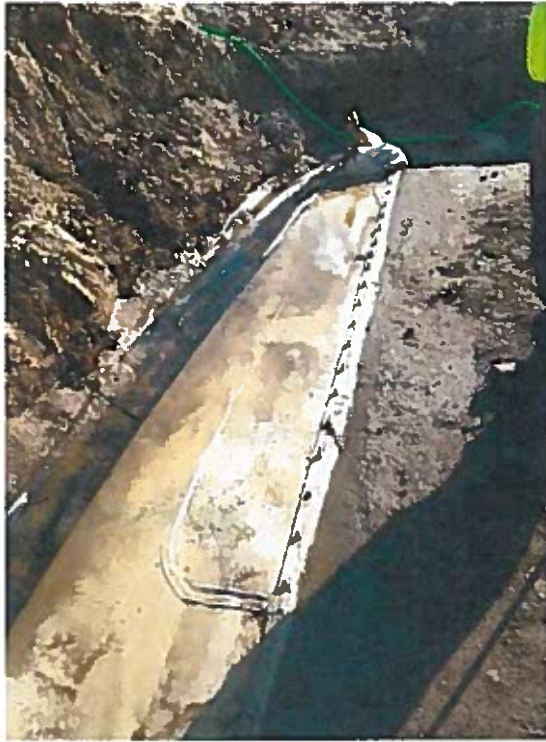
Damaged connection to batten strip on north side of weir wall, facing southwest
