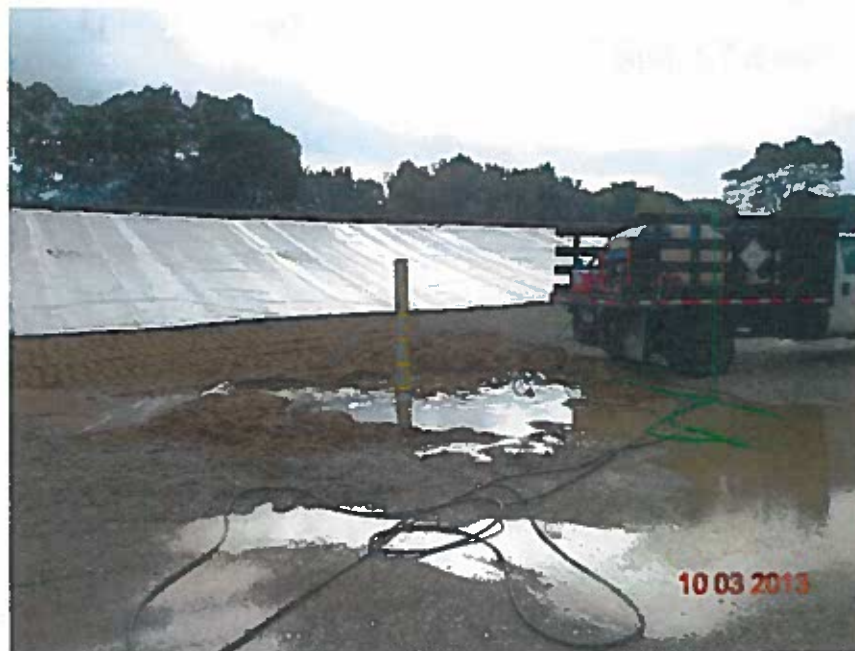
Pumping water from riser pole after the rain (looking southeast)
