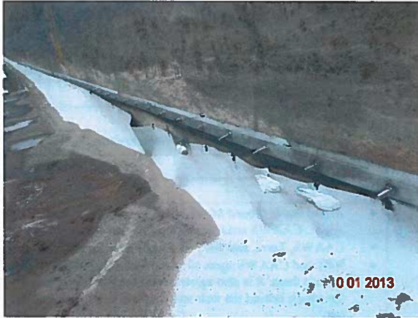
Section of the torn batten strip (looking southeast)
