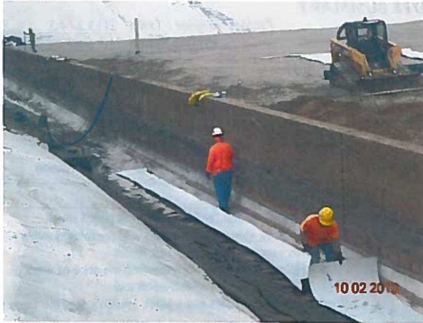
Geomembrane sections being added to the liner to provide slack for the transition between the basin floor and weir wall (looking southeast)
