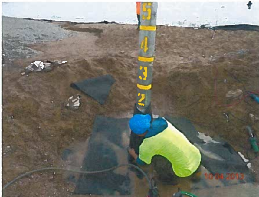
Installing the upper nonwoven geotextile over the geomembrane pipe boot (looking east)
