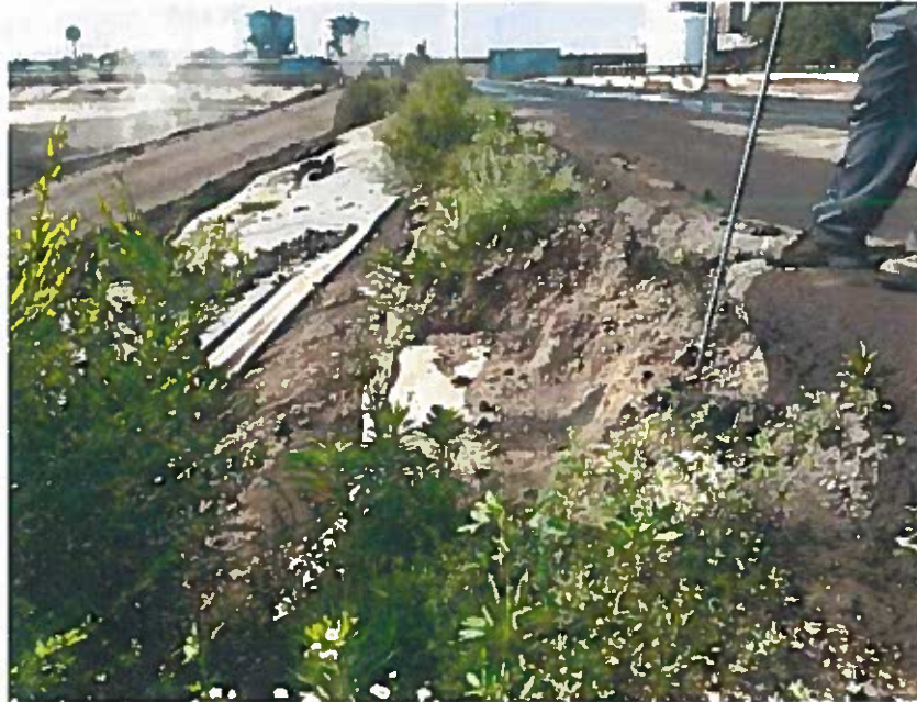
South-facing view of top of western slope, anchor trench will be constructed next to road, road material to be placed on top for transition to road
